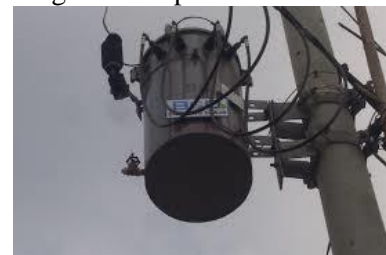
Gambar 2.2. Transformator Distribusi 1 Fasa ( https:// wordpress.com/ )
