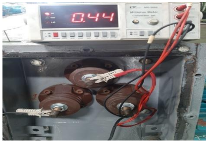
Gambar 4.6 Pengukuran DC Resistance Test
